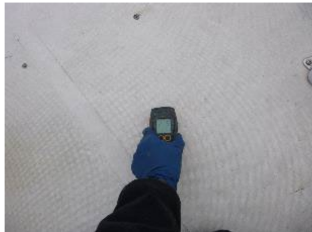
Elevated moisture in the hardtop. Meter reading 207.
