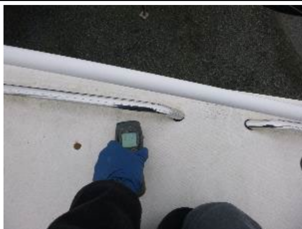
Elevated moisture in the hard top to port. Meter reading 202.
