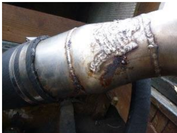
The repaired stainless-steel exhaust mixing elbow leaks.
