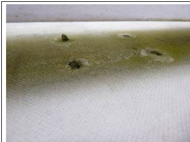
Poorly filled old fastener holes in the hardtop below the course board structure.
