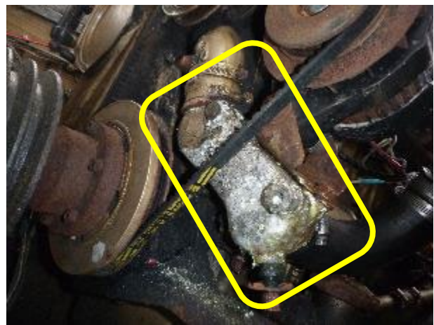
Corrosion and signs of antifreeze leaking to port of the circulating pump, below the alternator.
