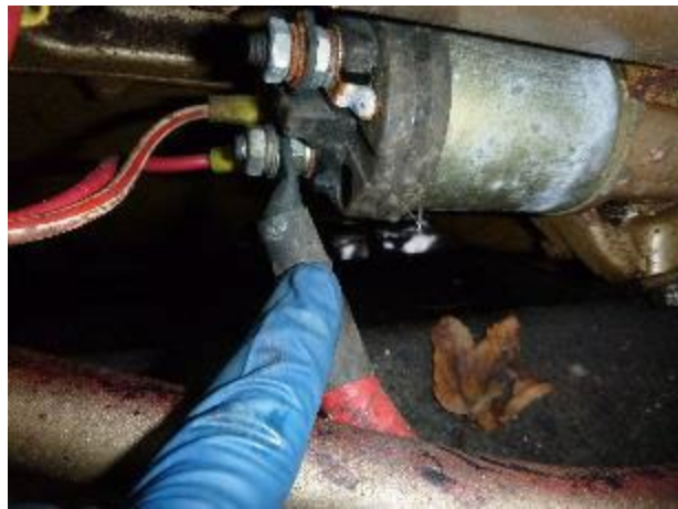
The engine starter positive cable connection needs a protective boot installed over it.
