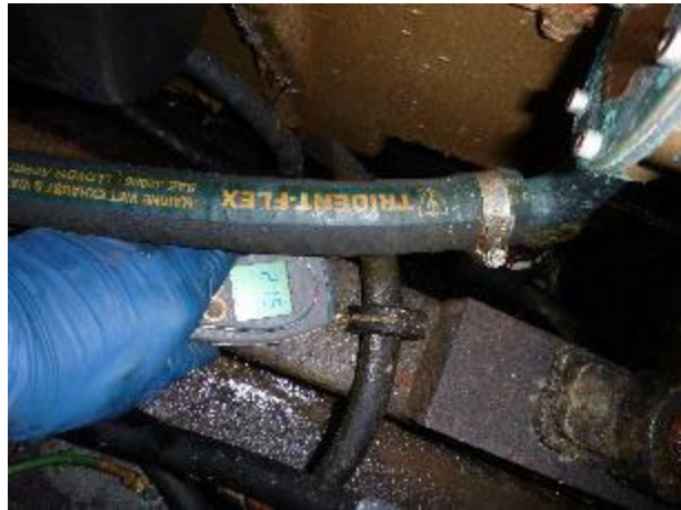
Elevated moisture in the starboard engine bed. Meter reading 215.
