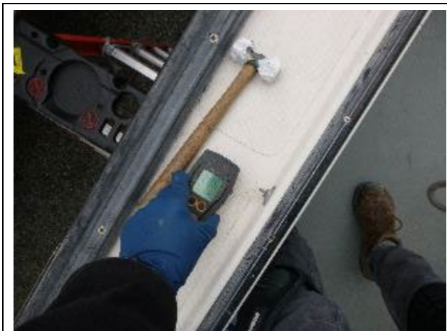
Elevated moisture in the starboard coaming top. Meter reading 215.
