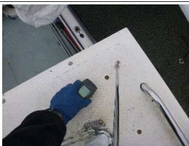
Elevated moisture in the hardtop, aft. Meter reading 212.
