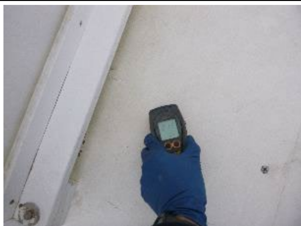
Elevated moisture in the middle of the hardtop. Meter reading 212.
