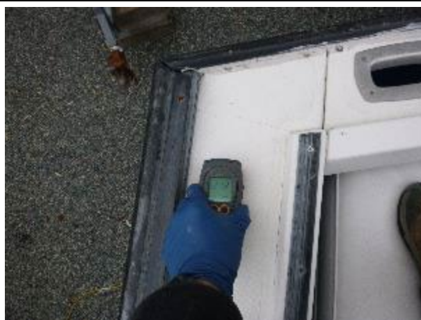
Elevated moisture in the starboard coaming top. Meter reading 212.
