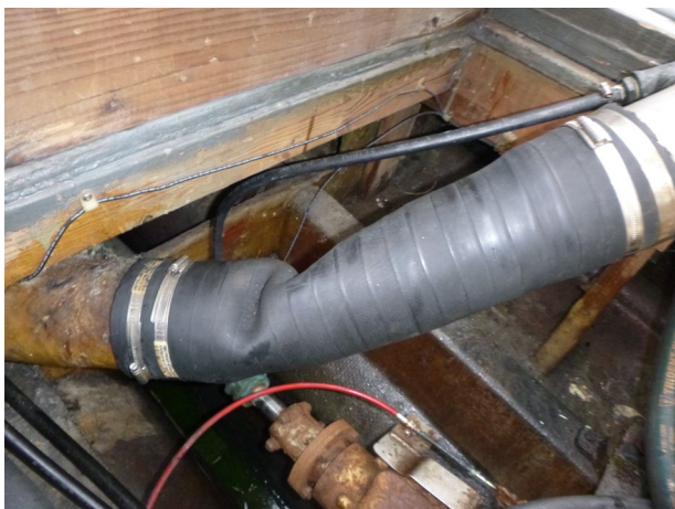
The exhaust hose is partially collapsed.
