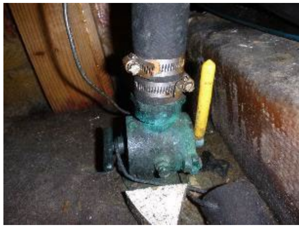
The engine intake through hull valve should be serviced and the rusted hose clamps replaced.
