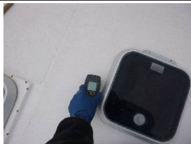
Elevated moisture in the forward trunk cabin deck. Meter reading 212.
