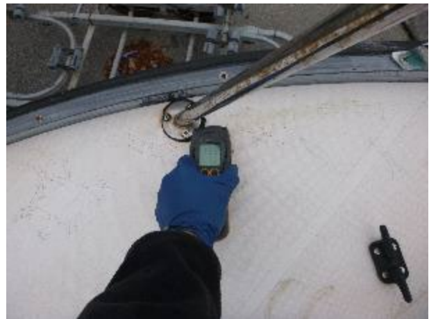
Elevated moisture in the foredeck. Meter reading 258.
