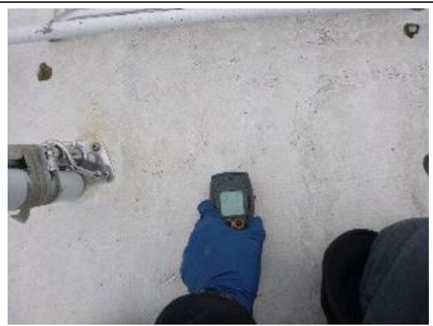
Elevated moisture in the hardtop to starboard. Meter reading 215.
