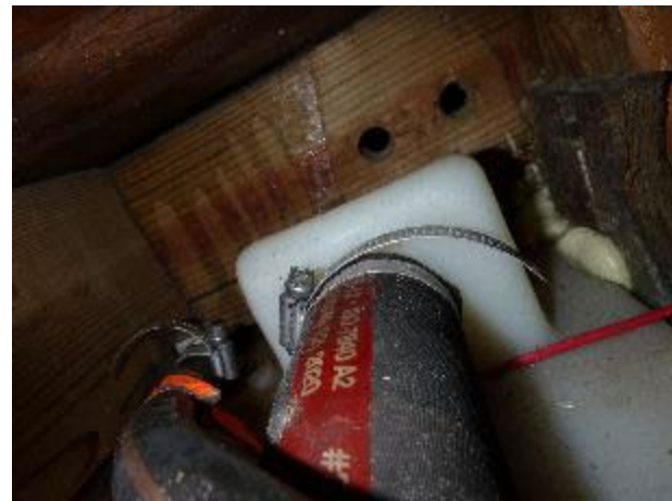
The fuel fill hose is not double hose clamped at the tank connection.
