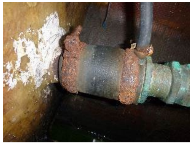
The stuffing box hose clamps are rusted, and the water injection hose clamp is broken.
