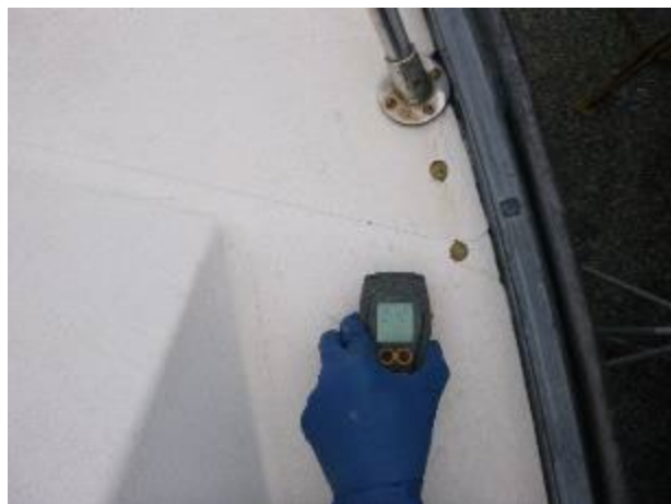
Elevated moisture in the starboard side deck. Meter reading 212.
