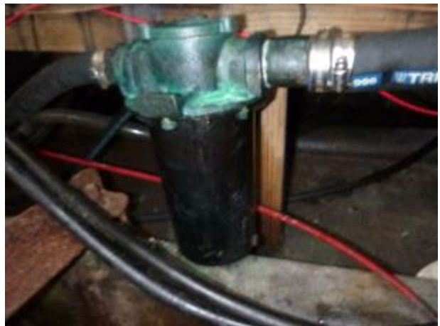
Then engine raw water strainer is missing its lower strap.
