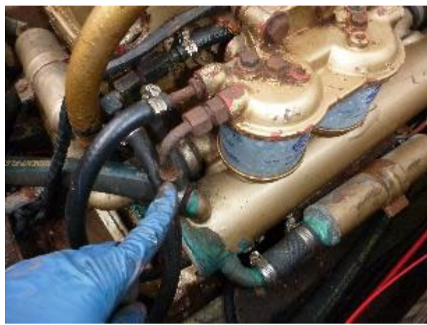
Rusted fuel fitting.
