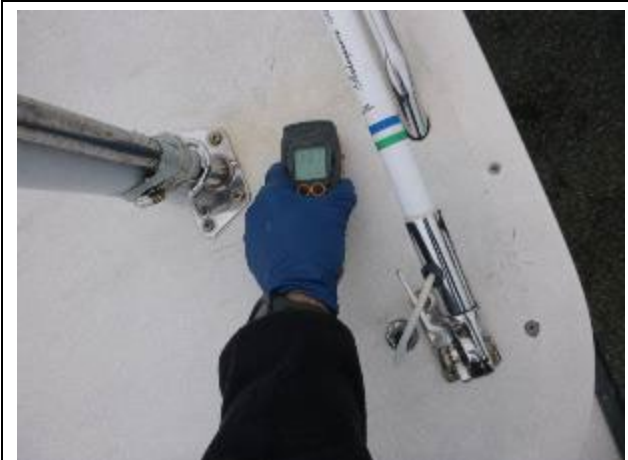
Elevated moisture in the hardtop, starboard forward. Meter reading 207.
