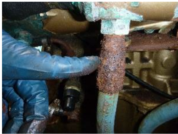
Rust and corrosion at the oil cooler to starboard.
