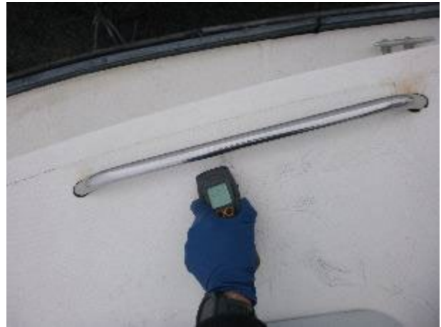
Elevated moisture in the starboard side of the forward trunk cabin. Meter reading 229.
