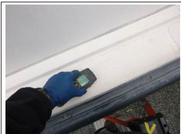
Elevated moisture in the port side deck. Meter reading 207.
