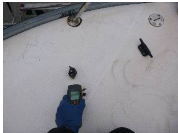
Elevated moisture in the foredeck. Meter reading 239.
