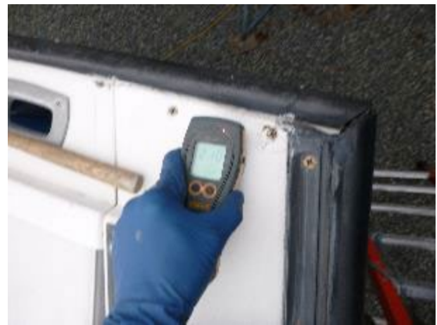
Elevated moisture in the aft end of the port coaming top. Meter reading 210.
