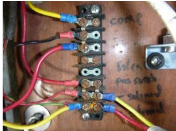
Rusted and corroded wiring terminal strip to adjacent to the horn compressor.
