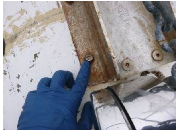
The anchor roller fasteners are not long enough to properly engage the nylon lock nuts.
