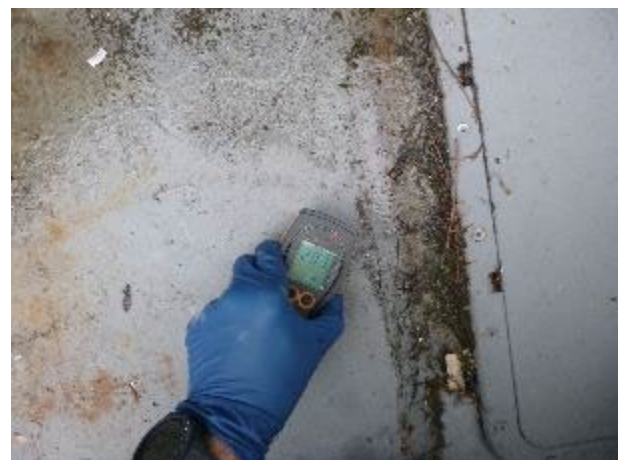
Elevated moisture in the aft cockpit sole. Meter reading 207.
