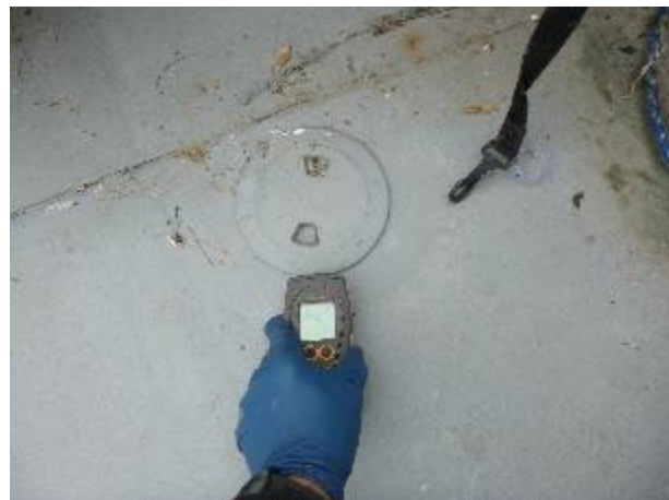
Elevated moisture in the cockpit sole to port. Meter reading 287.
