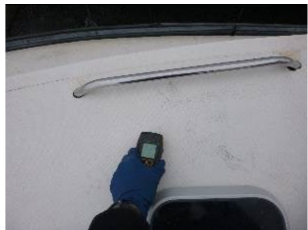
Elevated moisture in the starboard side of the forward trunk cabin. Meter reading 212.
