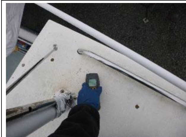
Elevated moisture in the hardtop, aft. Meter reading 210.
