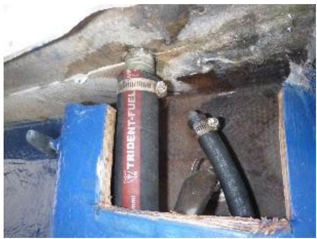
The fuel fill hose is not double hose clamped and is also loose on the deck fill spud. The fuel vent fitting is loose in the hull.
