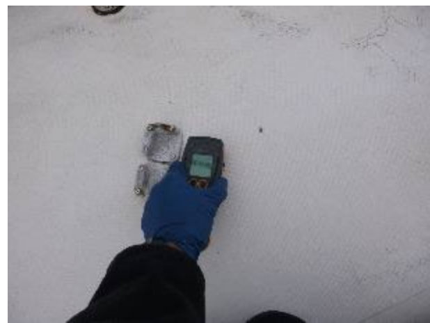
Elevated moisture in the foredeck. Meter reading 220.
