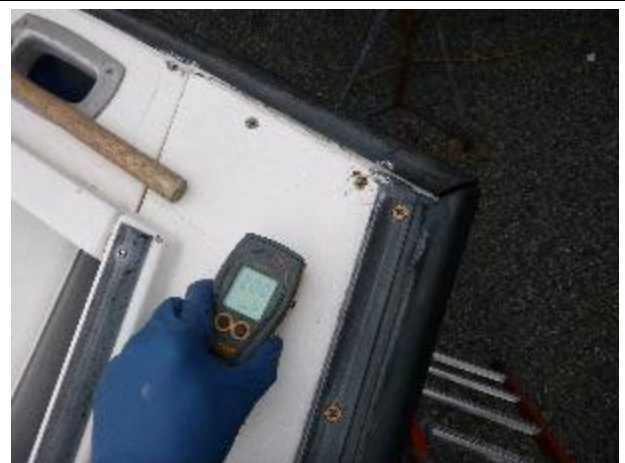
Elevated moisture in the port coaming top. Meter reading 200.
