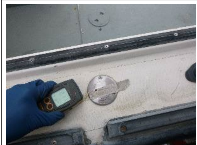
Elevated moisture in the port coaming top. Meter reading 217.
