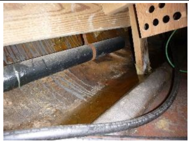
Standing water outboard of the starboard bilge stringer.
