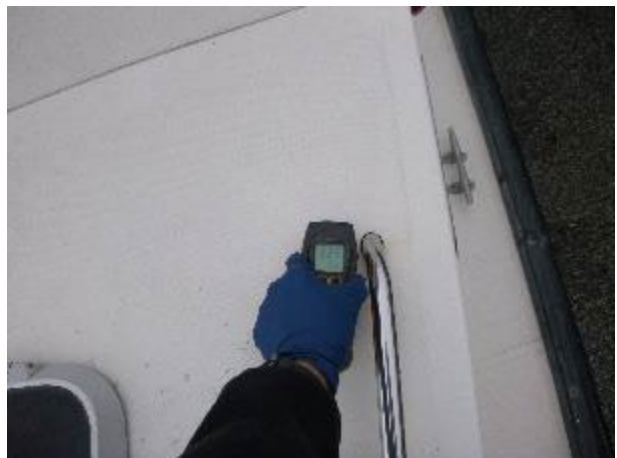
Elevated moisture in the port side top of the forward trunk cabin. Meter reading 229.
