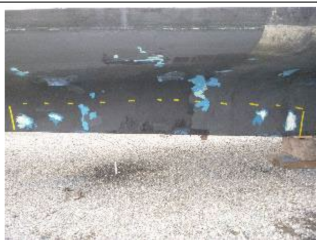
Yellow tape marking off area of gelcoat stress cracking the port amidships keel.
