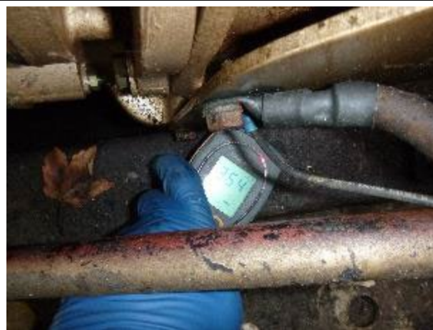
Elevated moisture in the port engine bed. Meter reading 354.
