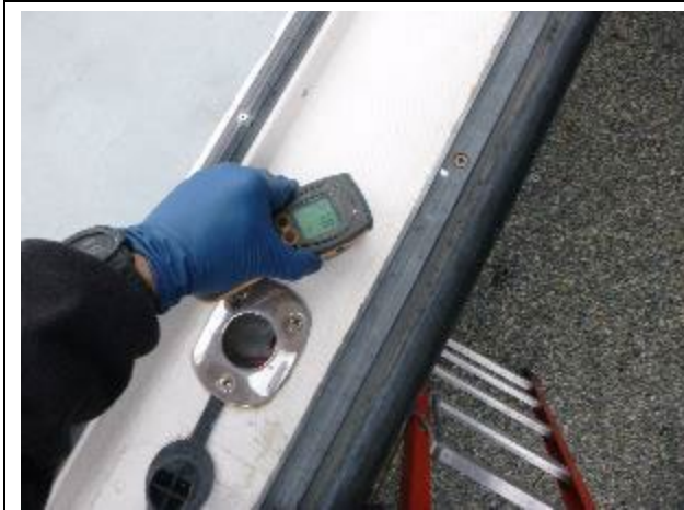
Elevated moisture in the port coaming top. Meter reading 218.
