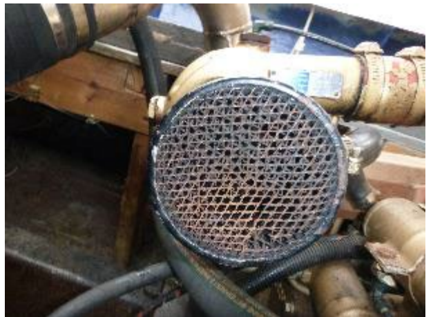
Air intake screen rusted through.
