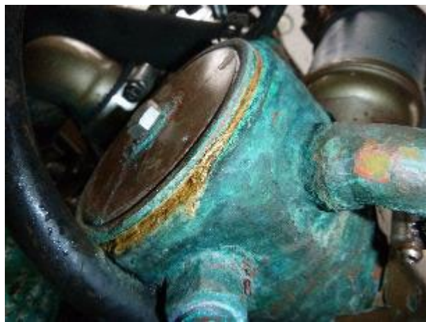
Engine heat exchanger corrosion.
