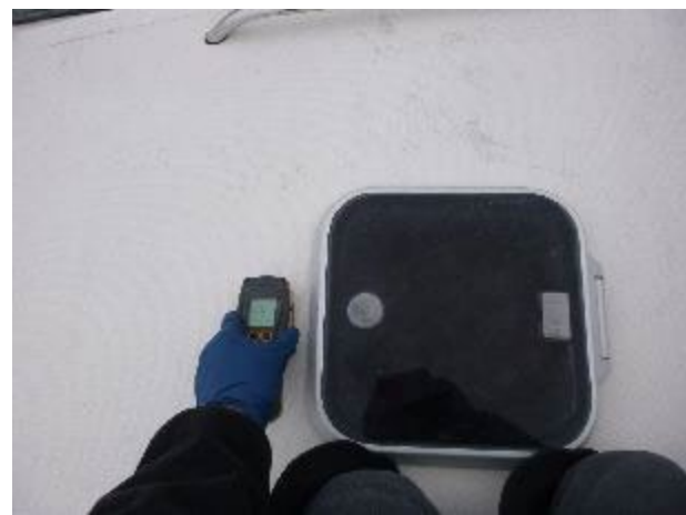
Elevated moisture in the starboard side of the forward trunk cabin. Meter reading 207.
