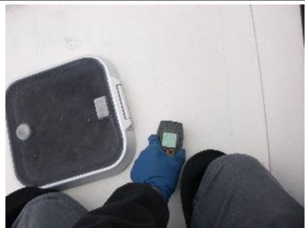
Elevated moisture in the starboard side of the forward trunk cabin. Meter reading 210.
