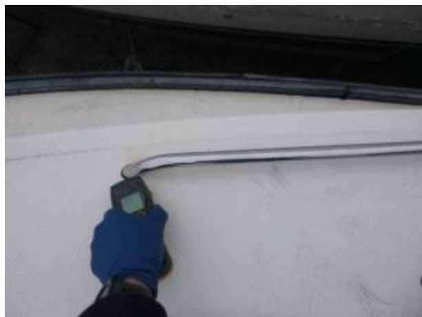
Elevated moisture in the starboard side of the forward trunk cabin. Meter reading 207.
