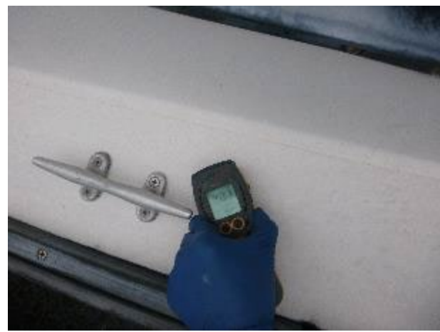
Elevated moisture in the starboard side deck. Meter reading 207.
