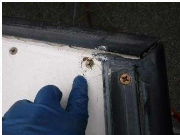
Pulled through transom coaming fastener.
