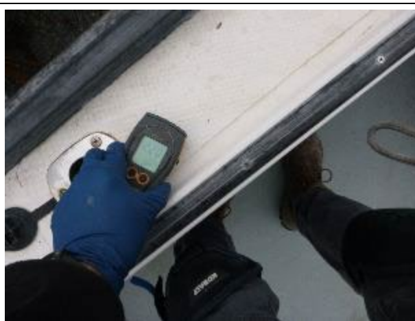
Elevated moisture in the starboard coaming top. Meter reading 220.
