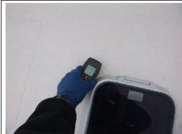
Elevated moisture in the forward trunk cabin deck. Meter reading 228.
