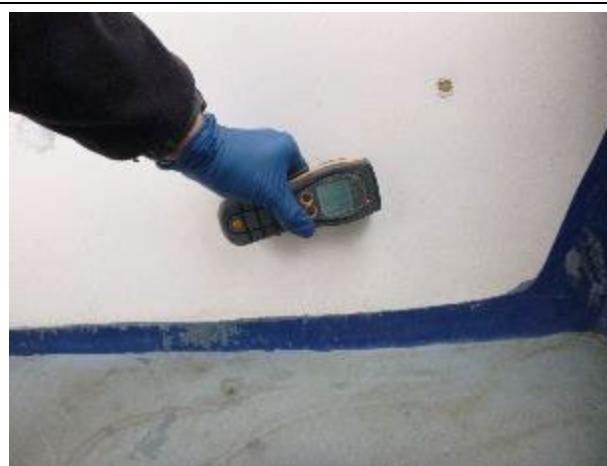
Elevated moisture in the main bulkhead below the helm to starboard. Meter reading 393.
