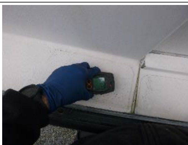
Elevated moisture in the port side deck. Meter reading 212.
