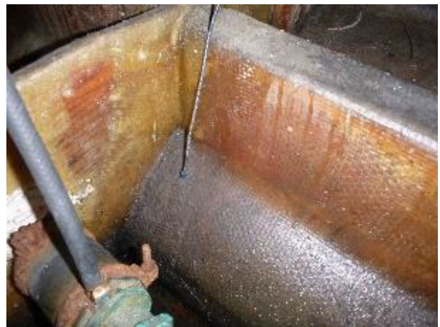
Abandoned ground wire in the port aft engine room bilge.
