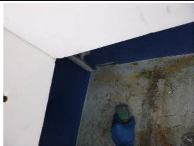
Elevated moisture in the aft cockpit sole. Meter reading 248.
