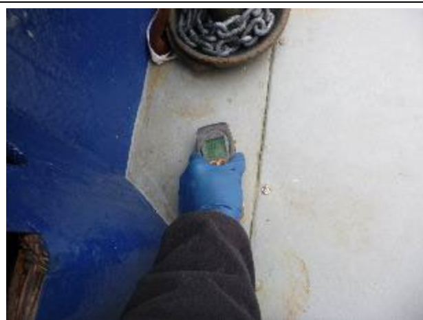
Elevated moisture in the cockpit sole to starboard. Meter reading 200.
