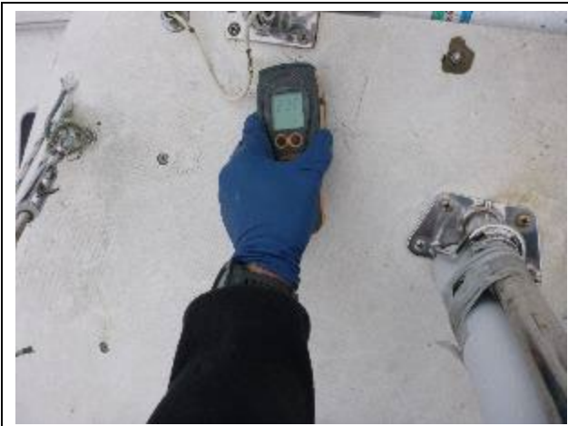
Elevated moisture in the hardtop to starboard. Meter reading 220.
