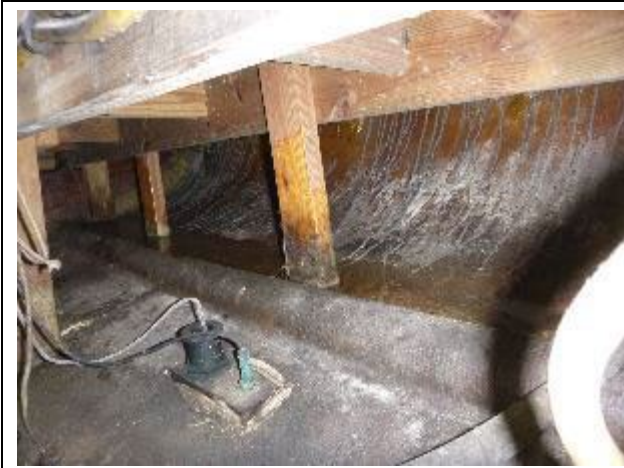
Standing water outboard of the port bilge stringer.
