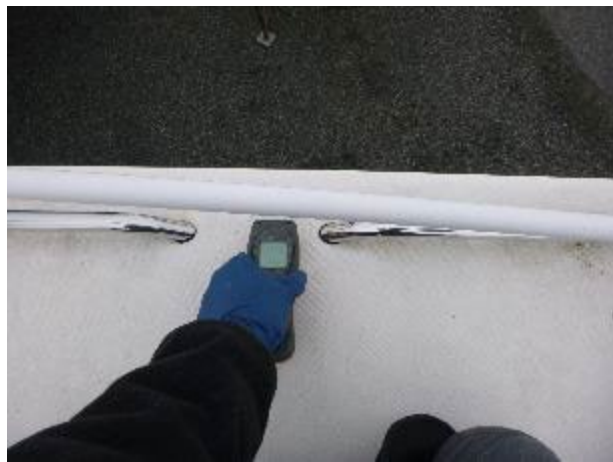
Elevated moisture in the hardtop to port. Meter reading 248.
