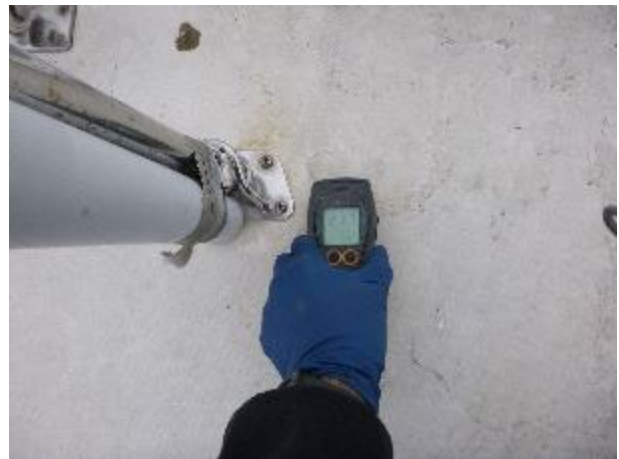
Elevated moisture in the hardtop. Meter reading 217.
