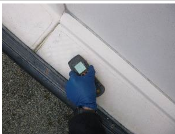
Elevated moisture in the port side deck. Meter reading 207.
