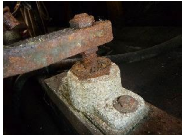
The port forward engine mount is deteriorated.
