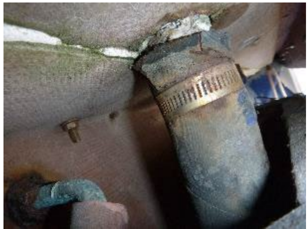
The fuel fill hose for the removed port fuel tank is deteriorated.
