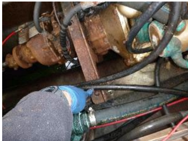
Fuel and steering lines should be chafe protected on the starboard aft engine mount bracket.
