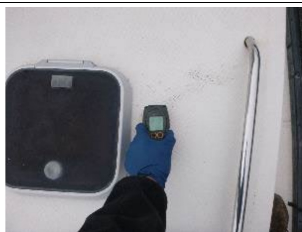
Elevated moisture in the port side top of the forward trunk cabin. Meter reading 212.
