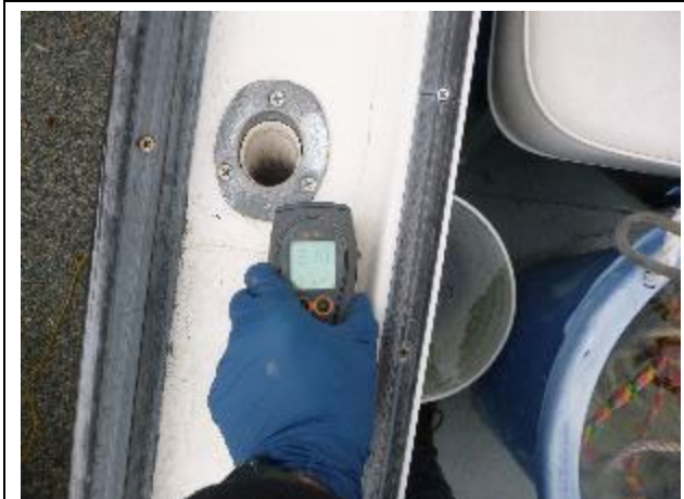
Elevated moisture in the starboard coaming top. Meter reading 210.
