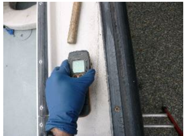
Elevated moisture in the port coaming top. Meter reading 220.
