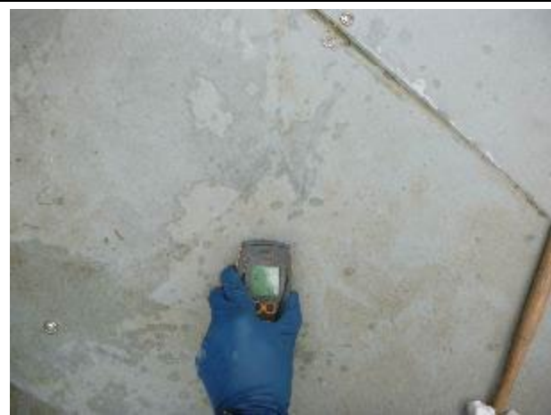
Elevated moisture in the aft cockpit sole. Meter reading 217.
