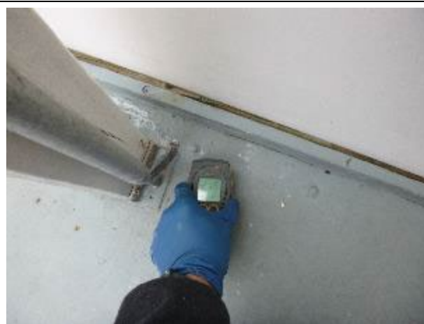
Elevated moisture in the cabinsole, forward to starboard. Meter reading 215.
