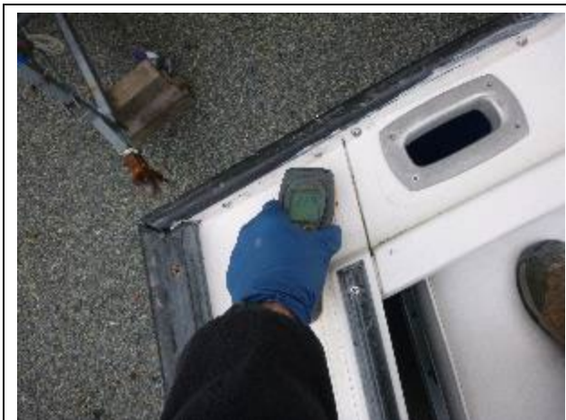
Elevated moisture in the starboard aft coaming top. Meter reading 229.
