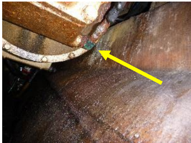
Oil line connection rust on the side of the transmission.
