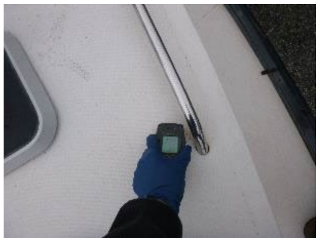
Elevated moisture in the port side top of the forward trunk cabin. Meter reading 220.
